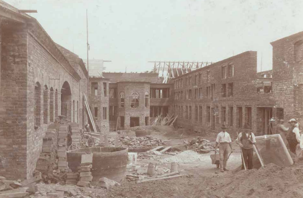
Kamenický Šenov, Elias Palme chandelier factory, house No. 686, view from the southwest into the courtyard of the main building during its construction; centre: main staircase; left: boiler and engine wing. Stanislav Kopecký's collection.
