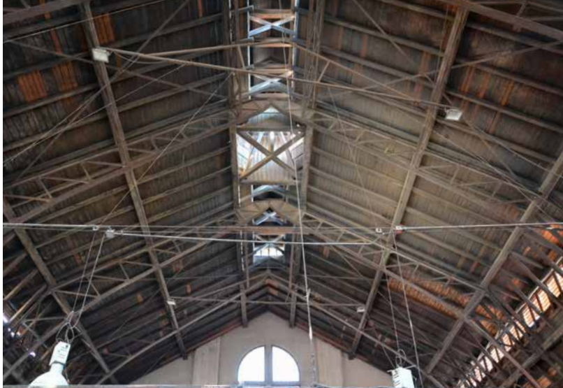
Kamenický Šenov, glassworks complex, house No. 687; view of the roof structure interior of the later glassworks hall in the direction of the southwest wall. Photo: author, 2019.
