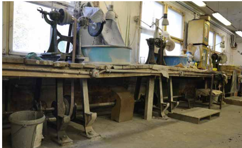
Nový Bor, Florahütte glassworks complex, house No. 399; grinding works with a detail of cutting lathes and the transmission system. Photo: author, 2018.
