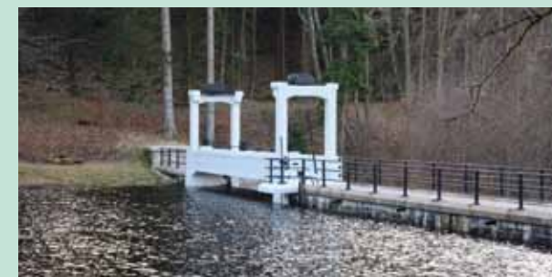
The dam of the levelling reservoir with an automatic valve stopper
