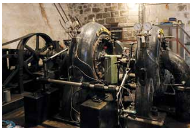
MVE II plant room with the Francis turbine
