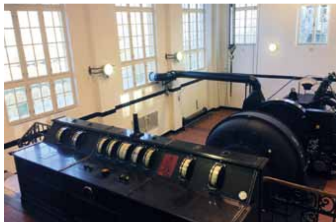
MVE I plant room with the Pelton wheel
