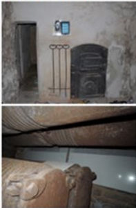
HEATING CHAMBER WITH CALORIFIER
