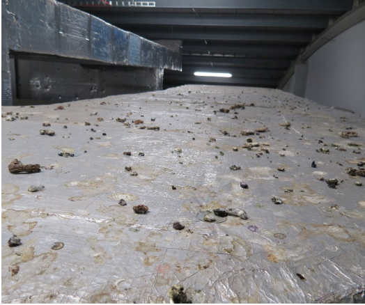
Fig. 5: Bird droppings after penetration of birds into the technical areas of MG depositories, providing sources for the development of microbiological or insect biologic activity or for direct aggressive effect on buildings or materials of cultural heritage.
